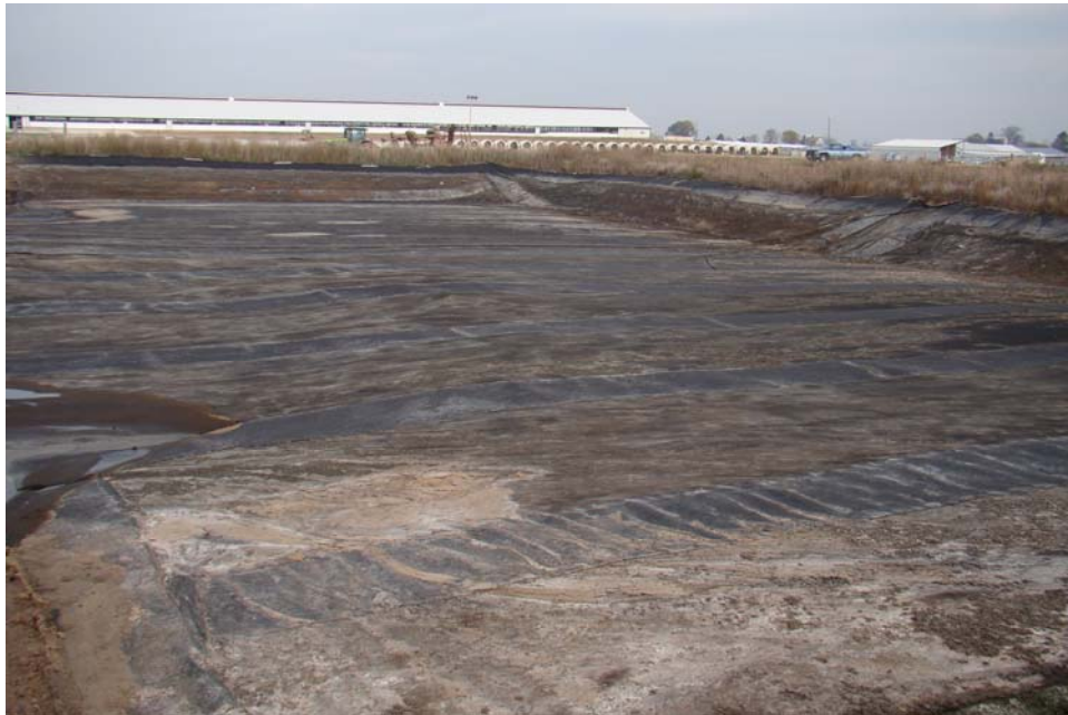
Figure 3.1 Permeable Cover on Lagoon #2, Kewaunee County Farm
