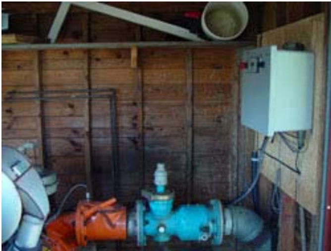
Control Box and Pump
