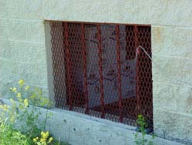
Metal Screen for Window Airflow/Vandals
