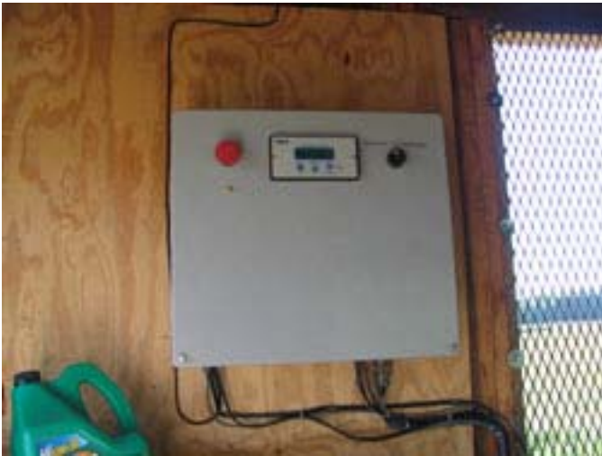
Controller in Pump House
