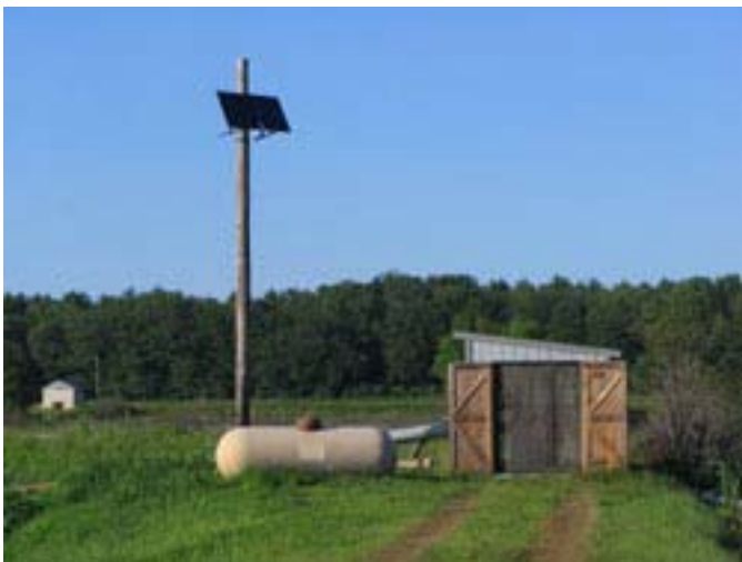
Solar Panel at Pump House
