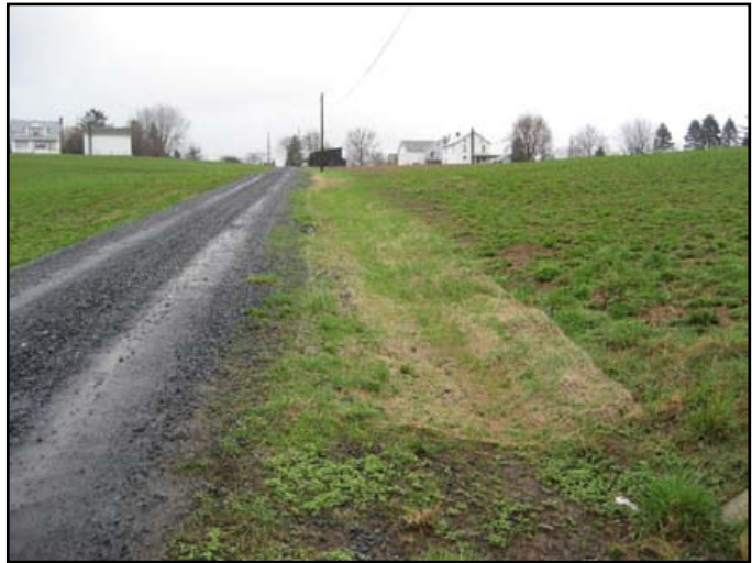
Figure 4.1: Grass is beginning to grow through the erosion matting in the newly constructed roadside swale.
