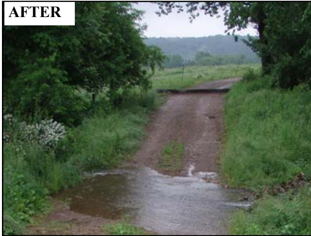
Figure 3: A conveyor belt diversion, installed before the ford crossing, insures runoff is diverted before it can reach the stream.
