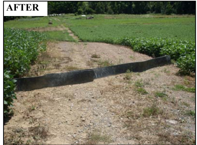
Figure 4.14: Three conveyor belt diversions can be seen in series on the hill slope leading to the stream at the tree line.
