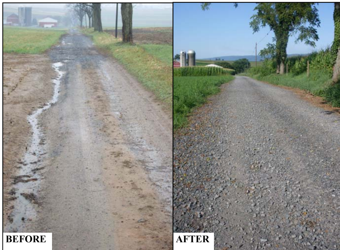
Figure 1&2: BEFORE the project, the entrenched farm lane collected field runoff and transported it down the road surface. Many practices were implemented to elevate the road, encourage infiltration, and insure that runoff could no longer use the road as a flow corridor.
