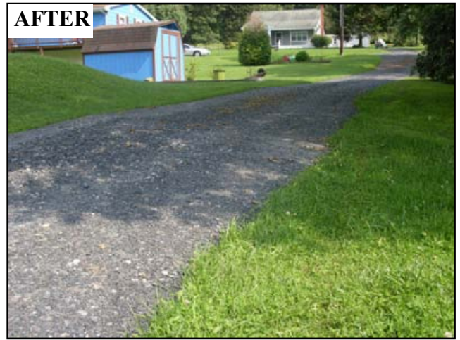
Figure 4.21: The improved road surface has a good shape and is resistant to traffic and erosion.
