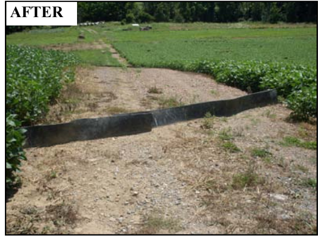
Figure 4: Three conveyor belt diversions can be seen in series on the hill slope leading to the stream at the tree line.
