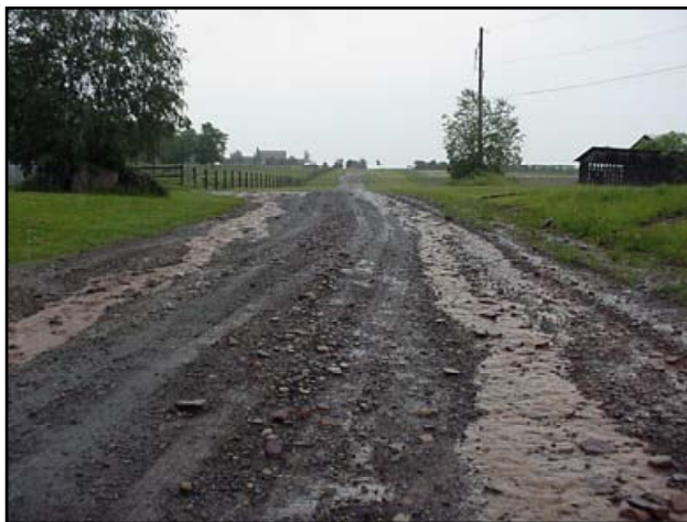
NO GRADE BREAK – Water flows on road causing excess erosion and aggregate loss.
