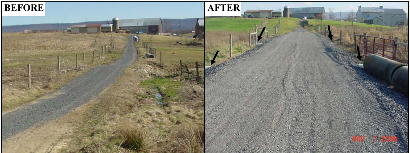
Figure 4.4: This is the wetland stream crossing on the Goss Farm. Notice that BEFORE, water is dammed up against the right side of the road and funneled through a single pipe. The AFTER picture shows the French mattress. White pipes are visible and highlighted with black arrows. Notice also that the road's "lowpoint" has been moved away from the stream so runoff is forced to leave the road before nearing the channel
