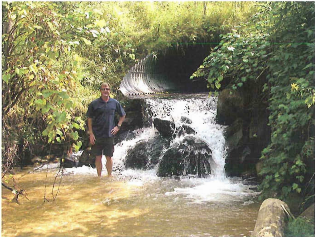
Perched culvert on Silver Creek completely blocking aquatic species passage approximately 300 yards from confluence with Pine River.
