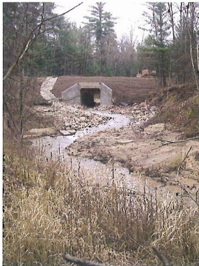
The completed structure includes paved approaches, runoff controls, and a clear span of the stream channel with virtually unlimited space for stream flow beneath the structure.
