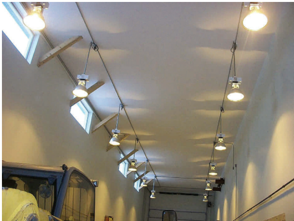
Truck Bay Lighting
