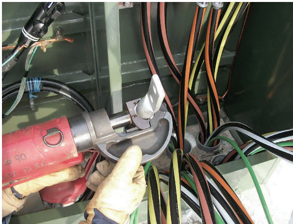
Generator Building Transformer Landing Cable
