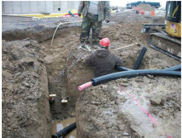
Natural Gas Piping
