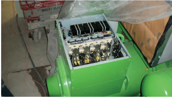
Generator Electrical Connector
