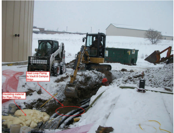
Yard piping—heat loops to vault & buildings
