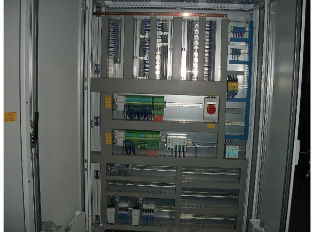
Control Panel right Side
