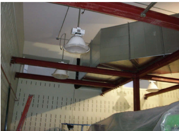
Generator room makeup air duct system & lighting
