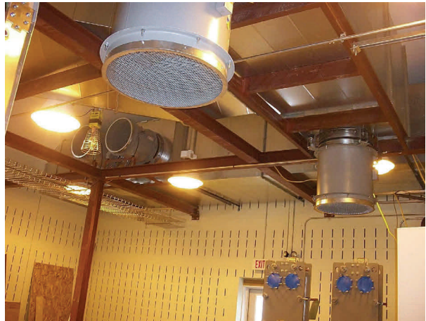
Generator Room Lighting
