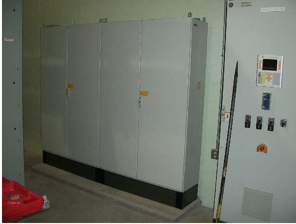
Control Panel Electrical Room
