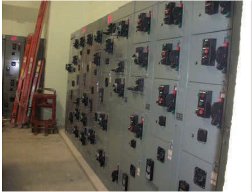
Control Panel Electrical Room
