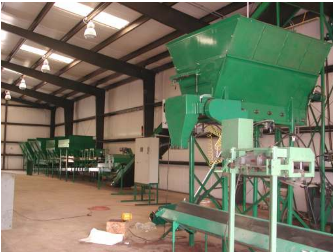
Mixing and Bagging Equipment Line.
