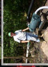
Figure 3. Heck Davis with new electric irrigation pump.
