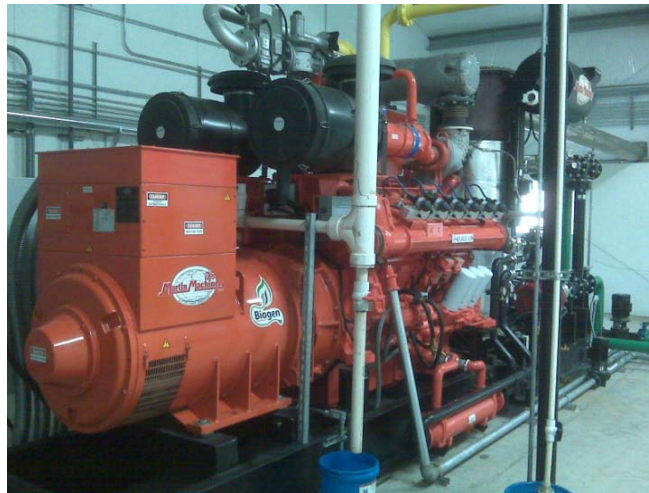
Figure 10. 450 KW generator run on methane to produce electricity.
