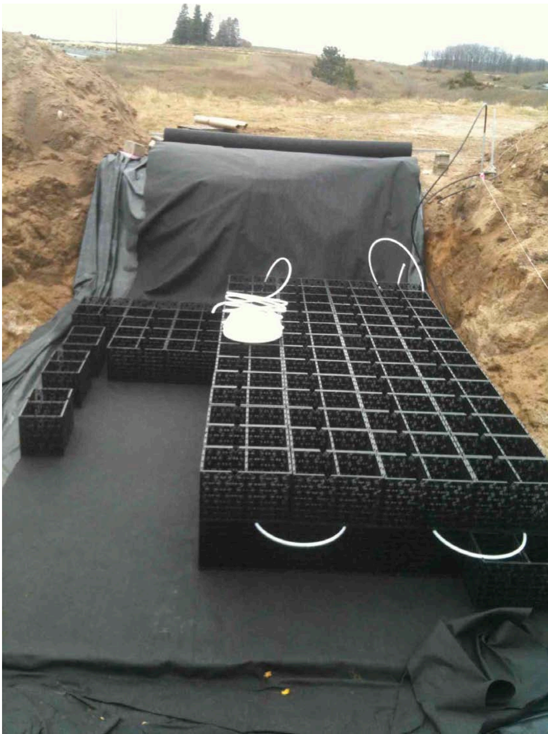
Figure 1.1 Water Conservation tank assembly
