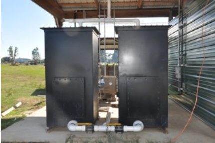
Biogas Scrubbers (remove H 2 S)
