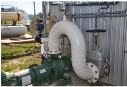
Poultry manure slurry inlet into the digester
