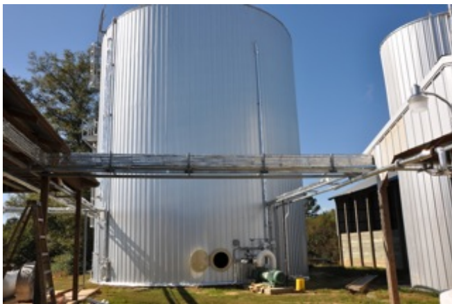
Upright insulated digester tank
