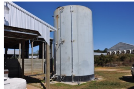
Fresh water storage tank
