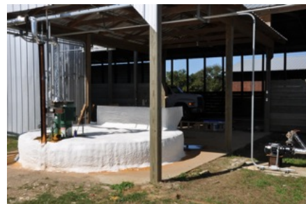
Insulated slurry pre-mix tank
