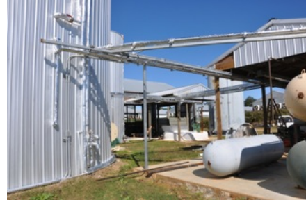
Digester tank connections for external heat and effluent
