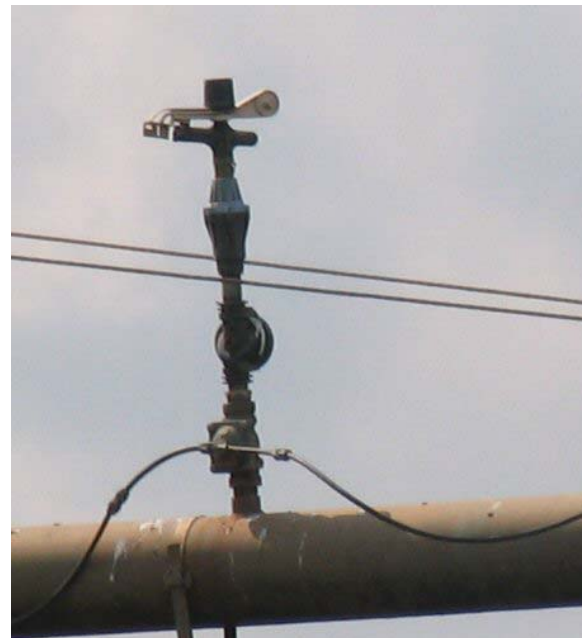
Figure 3. Control valve for CP sprinkler under VRI control.
