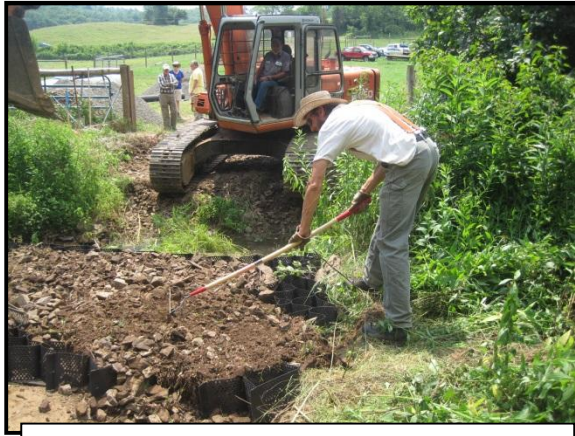
Hillsville, Virginia: Geo-web™ cellular confinement system to be used as a minimalist approach to hardening a portable timber bridge abutment.
