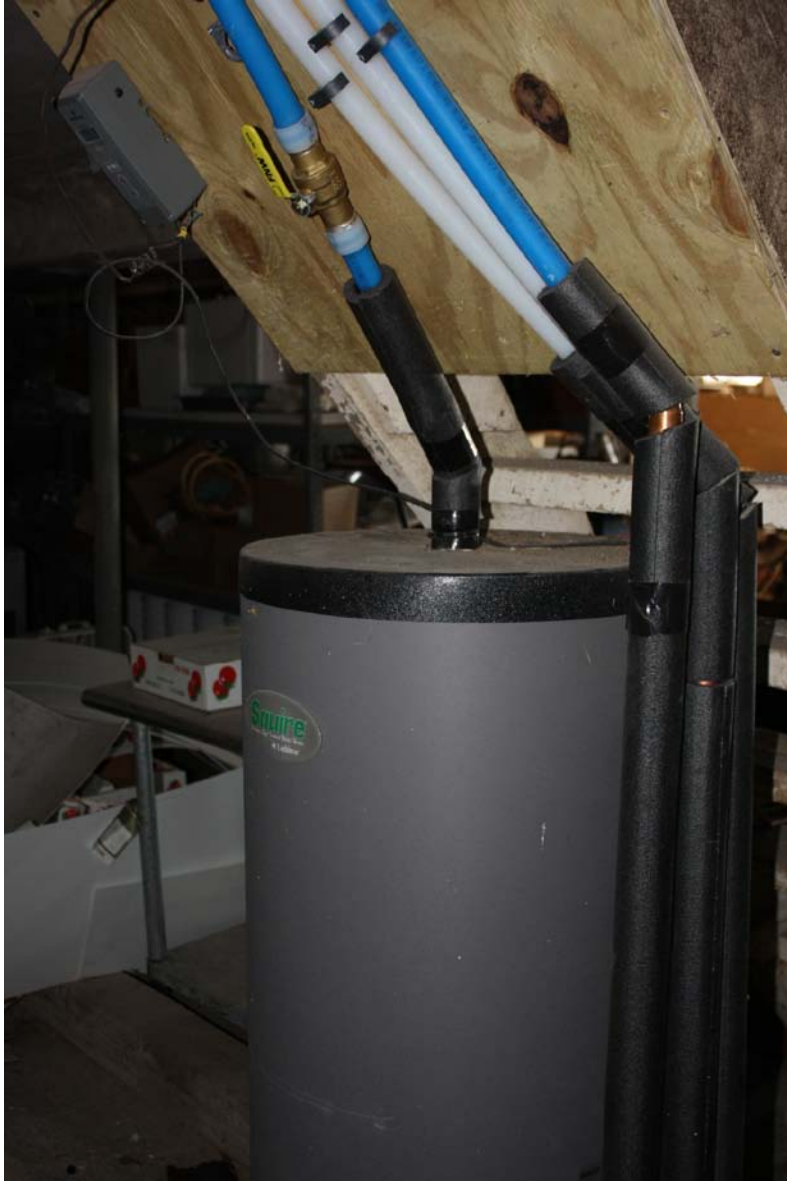
Figure 1.5 Chilled water heat exchanger tank for field heat removal system.
