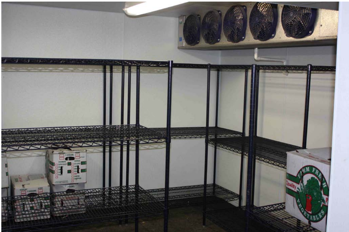
Figure 1.1; Interior of Geothermal Walk in Produce Cooler
