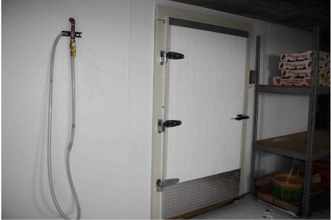
Figure 1.2; Exterior of Geothermal Walk In Produce Cooler
