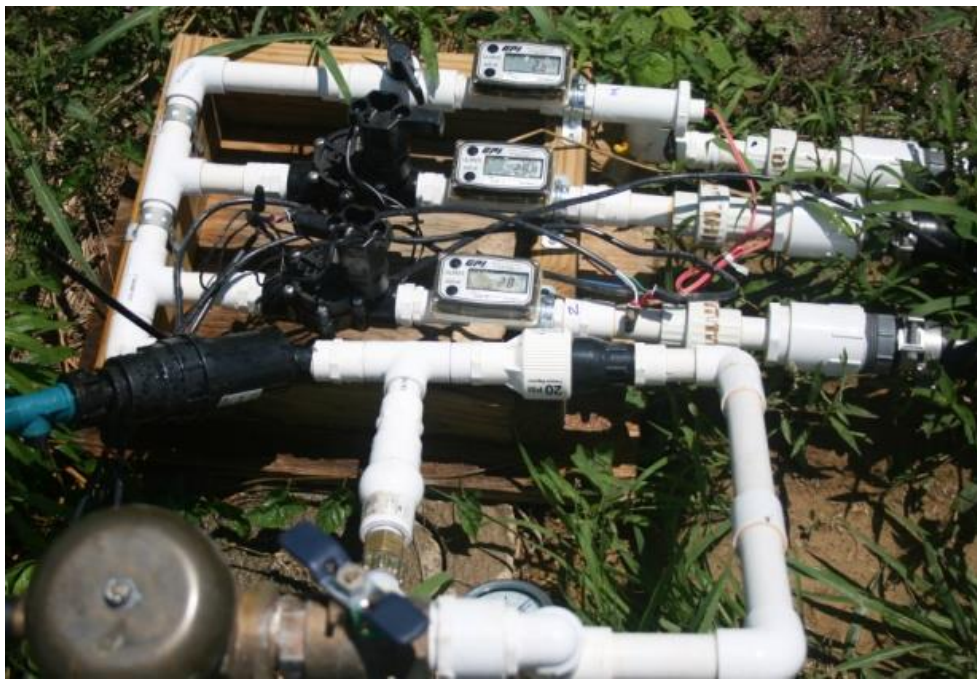
Figure 14: Control Manifold at D&F Farms
