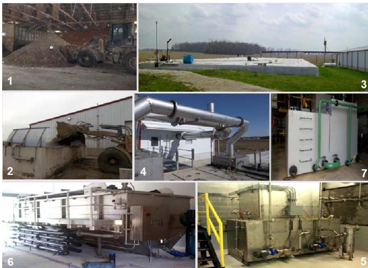
Figure 10: Wenning Poultry ( 150,000 \text{ gallons day}^{-1} )—(1) poultry solids collection; (2) mixing with return/dilution water, (3) anaerobic digestion (CHP); (4) ammonia stripping; (5) ammonia sulfate production; (6) DAF/P solids separation; and (7) \text{H}_2\text{S} removal from biogas
