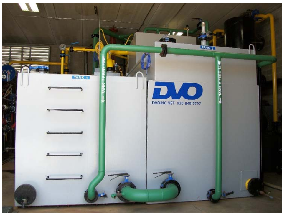
Figure 12: Dallmann Dairy H 2 S scrubbing unit (67,000 gallons day -1 )
