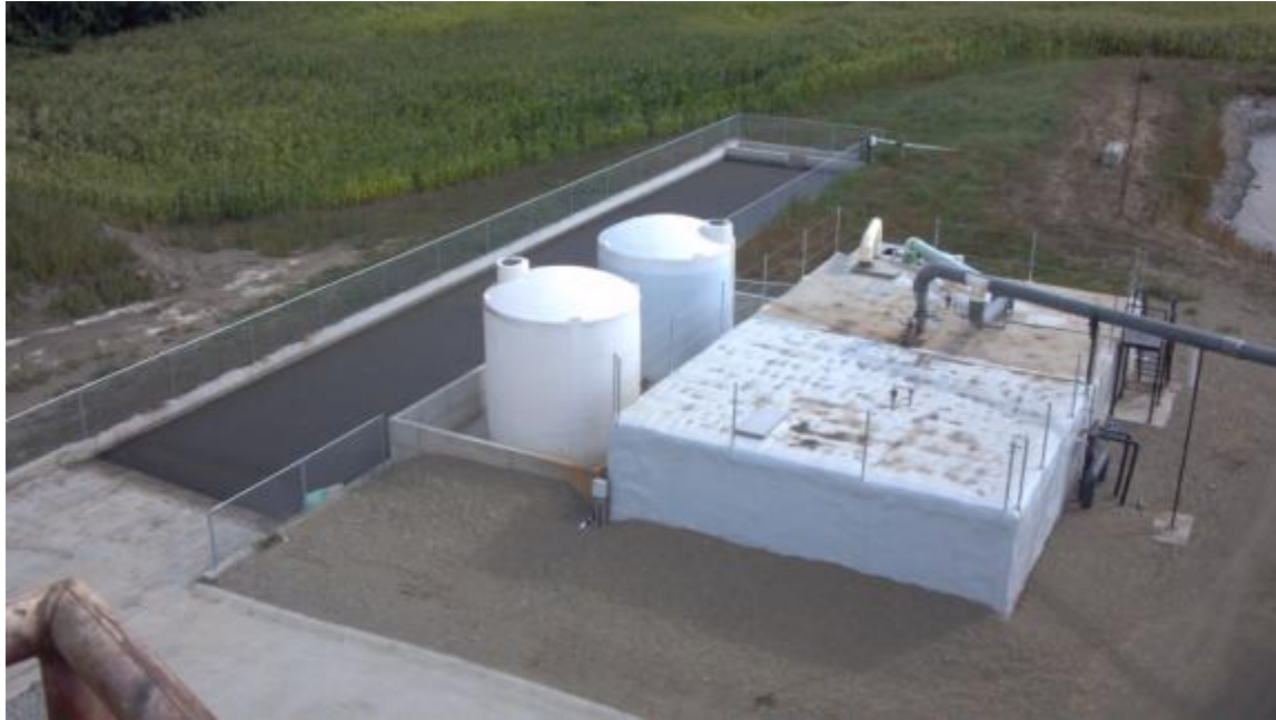
Figure 2. Commercial-scale P and N nutrient recovery facility integrated with dairy anaerobic digester, Lynden, WA (AD facility is not shown in photo).
