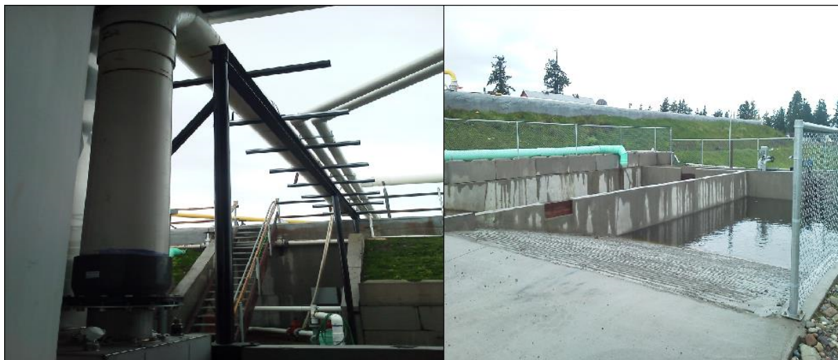
Figure 11: Rainier Biogas (85,000 gallons day -1 )
