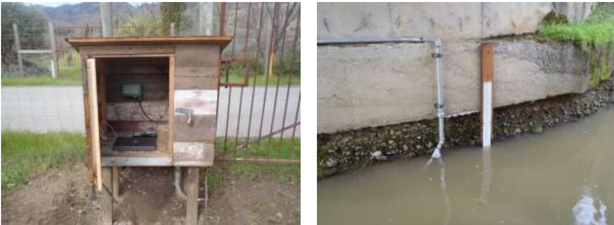
Figure 5c. Bubbler gage Installed in the McNab Creek Watershed with staff gage.
