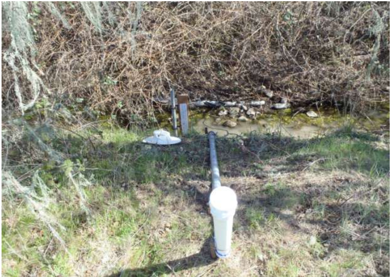
Figure 14: Pressure transducer in pipe housing with adjacent outside staff gage
