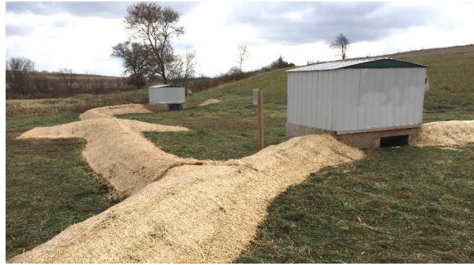
Figure 10. Wisconsin in-line installation with soil berms to prevent run-on between stations. The prototype (right) was positioned upstream of the conventional station (left)
