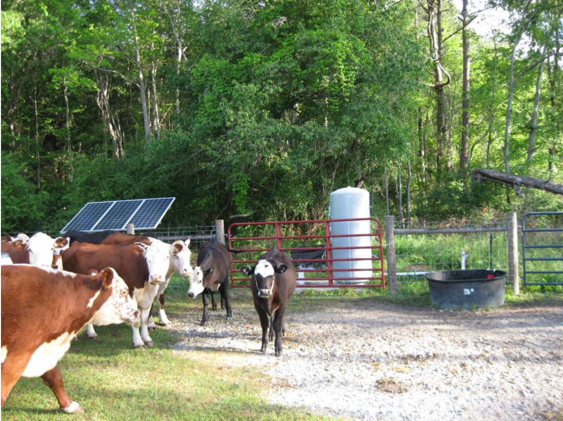
Figure 4. Livestock watering system where solar was used to lift water with a high total dynamic head. This system includes a pressurized tank and pushes water to multiple pastures on the farm.
