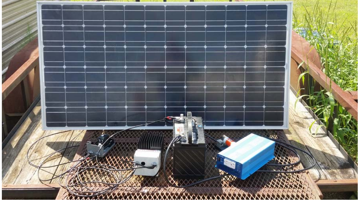
Figure 3. Set-up of the typical system used to convert solar power to AC power. This includes a solar panel, disconnect box, charge controller, fuse, battery and inverter.
