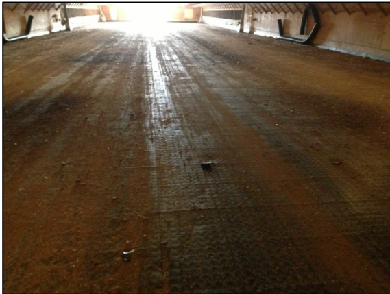
Picture 7. Broken tiles
