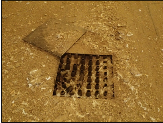
Picture 11. Damaged support cones
