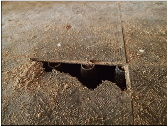
Picture 9. Broken tiles
