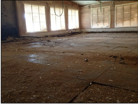
Picture 5. Raise edges and broken tiles.
