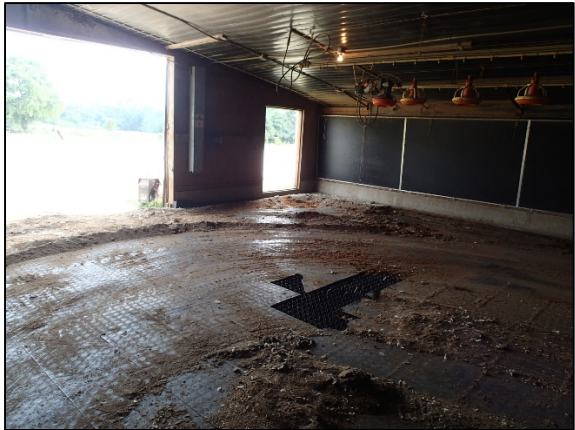
Picture 10. Broken tiles
