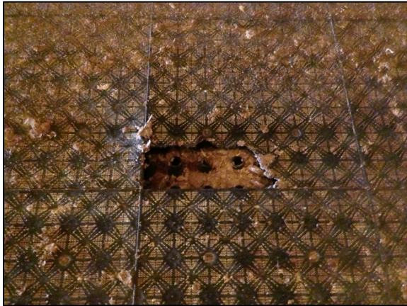
Picture 8. Broken tiles
