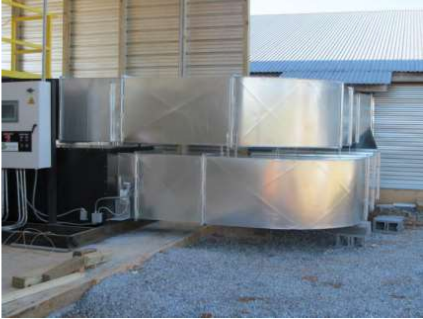
Duct work from the combustion unit to the poultry house
