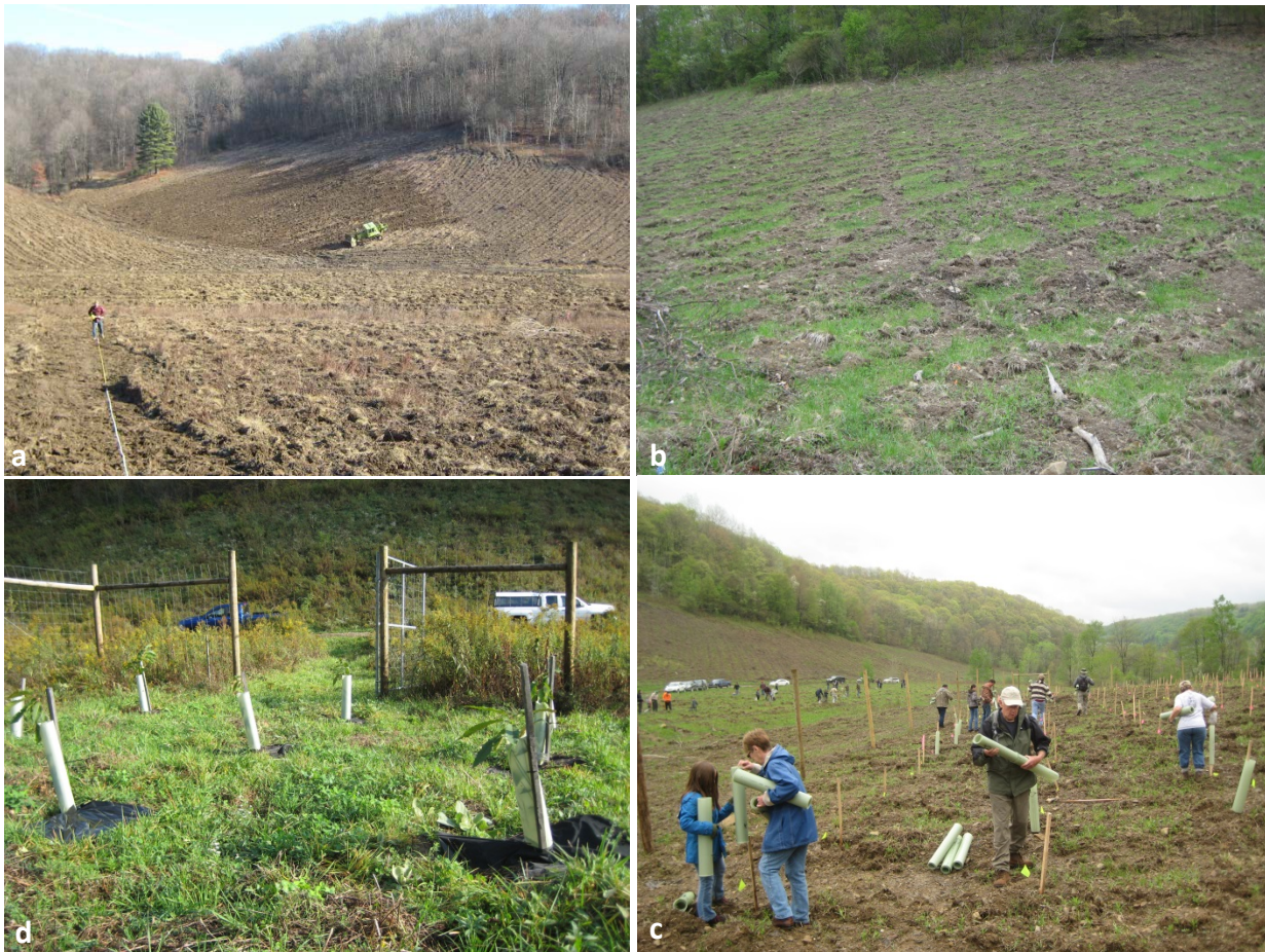
Clockwise from top left: a) A bulldozer cross-rips slopes while the progeny test area is being laid out. b) The diamond-pattern that results from cross-ripping on slopes. c) Volunteers distribute tree shelters before planting the progeny test. d) Seedlings emerging from shelters, two years after planting.
