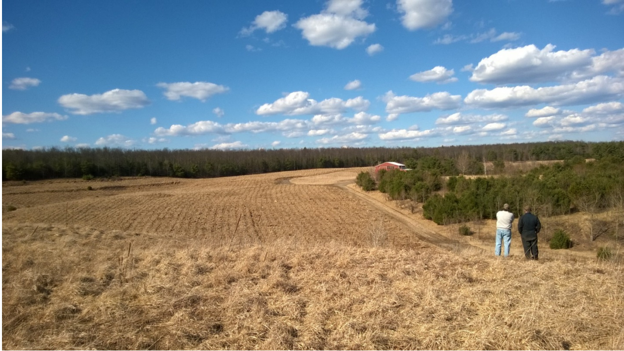
The landowner and the bulldozer operator inspect the reforestation area after cross-ripping in Clinton County, Pennsylvania. (photo by N. Hall)
