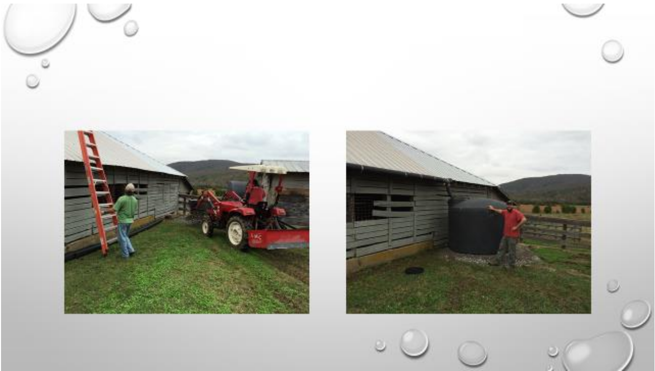
Graham Farm Rain Catch System, Estill Fork, Al. FSA Farm# 2109
