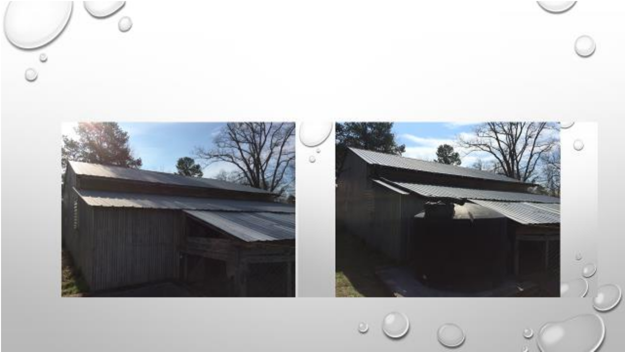
Before and after pics of installed system.
