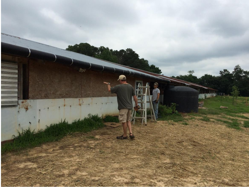
Gavin Moy Rain Catch System, Horton, Al 35980 FSA Farm# 2489
