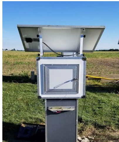
Figure 9. Modified equipment enclosure mounted to the drainage control structure
