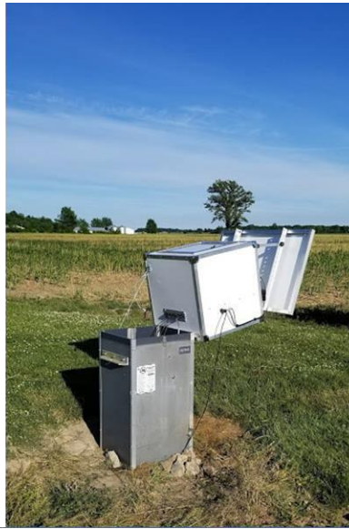
Figure 10. Hinged enclosure allows easy access to drainage control structure.
