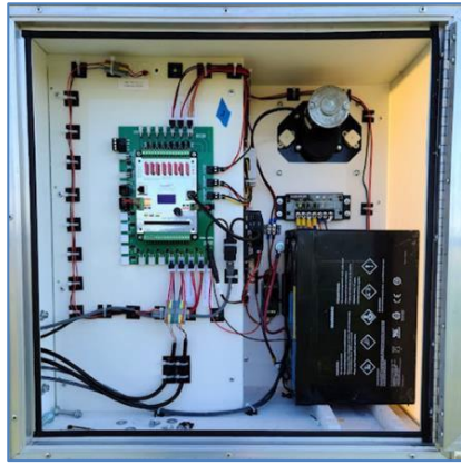
Figure 12. Rear door of provides excellent access to electrical-mechanical systems provides excellent access to electrical-mechanical systems.
