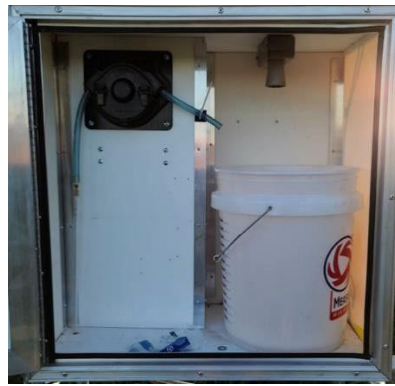
Figure 13. Front door of enclosure provides access to sample pump and sample container.
